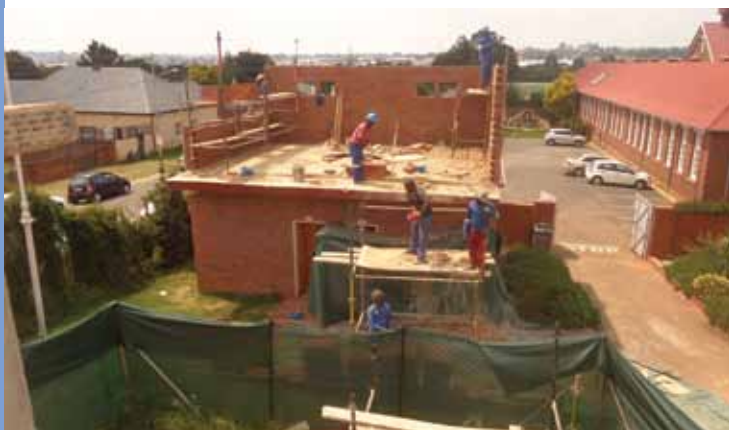
Beginning the second floor of the ablutions block, a necessary part of the school extension
