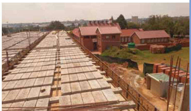
View of the preparation of the second slab of Bosco House for the third floor, looking north to Sarto House and the priory
