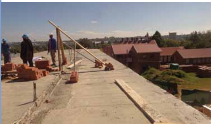
Looking north on the top of the third floor slab just poured to the priory. Work on the new classrooms started the very next day
