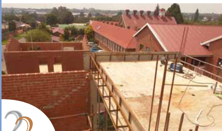
Top of stair case well, looking north to the ablution block and the priory
