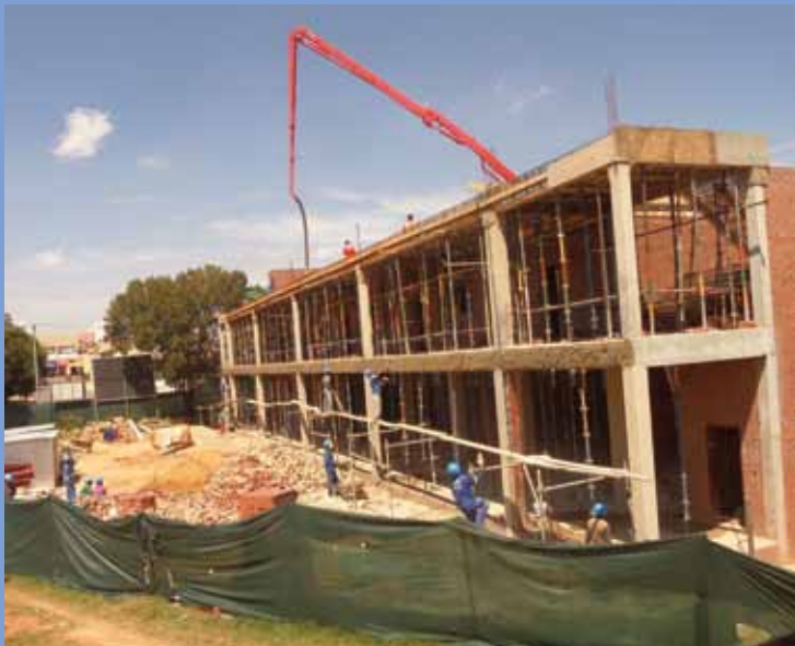
The cement pump used to pump cement from the ground to pour the top floor slab on March 9
